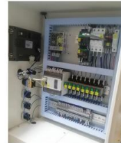
Electrical Control Cabinet
